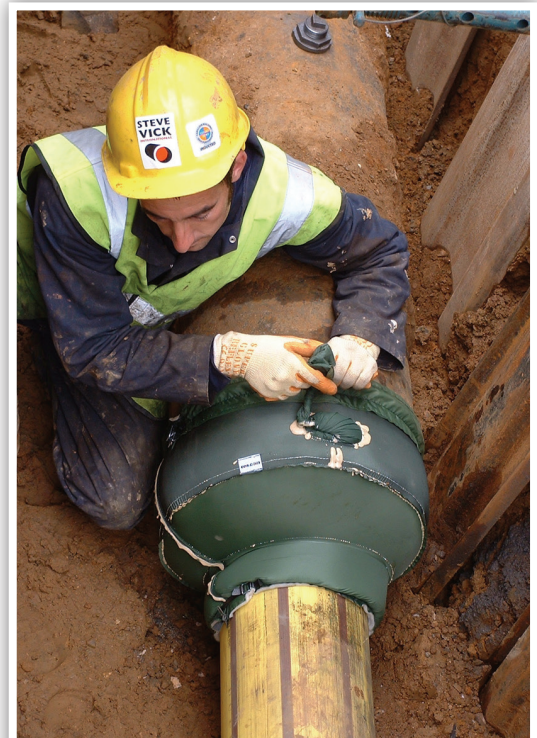
ENDSEAL™ being fitted to an inserted main (225mm PE into 16" cast iron main)
