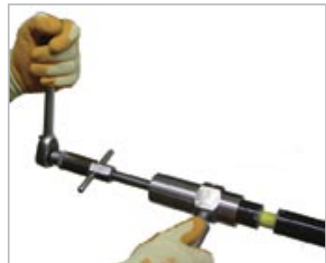
Diagram 4: The severed section of metallic pie and cured foam sealant is pulled away
