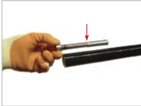
Diagram 1: Using the groove on the Gauging Bar as a guide, the service pipe is scored at the cutting point
