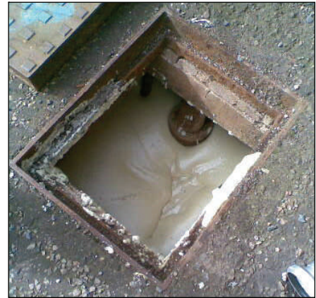
A redundant manhole chamber filled with expanding resin foam. Chapelcross Power Station
