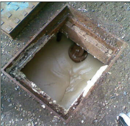
One of the 43 redundant chambers which were filled, remotely, using expanding polyurethane foam
