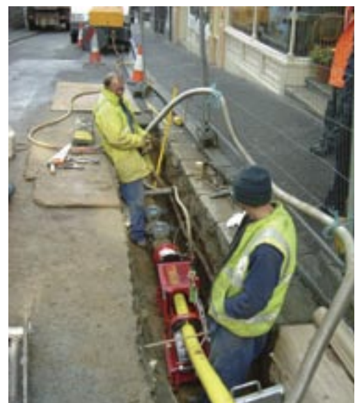
A member of our Special Contract Service team provided on-site technical support during this low pressure live mains insertion project.
