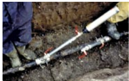
On medium pressure services, the FOAMBAG™ is introduced under 'no gas' conditions using a special angled tee
