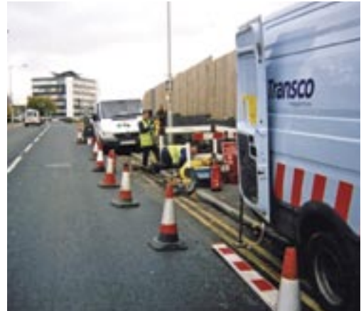
A remote stub end abandonment being carried out live in a sensitive traffic area close to a hospital and police station
